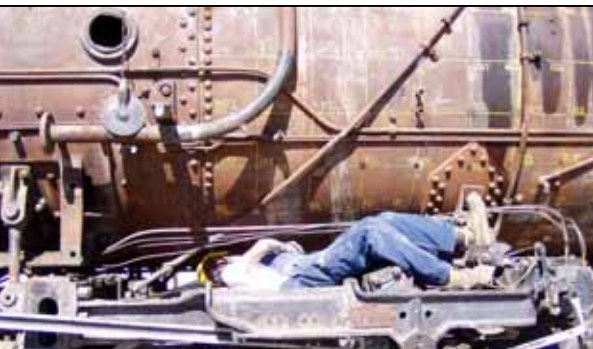
Zack Blea begins to squeeze into place atop the frame of 2926 to begin ultrasound measurements of the bottom of the boiler. Size, reluctant muscles and stiff joints keep most members from even thinking about such maneuvers.
